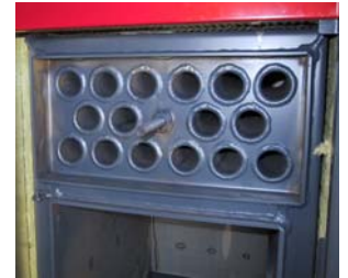
Boiler shown with dismantled cleaning door to flue tubes
