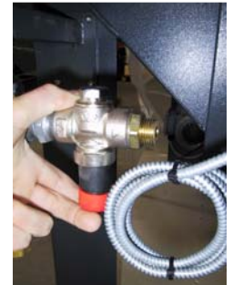
Sprinkler valve with dismounted hose
